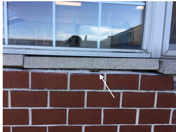
Embedded anchor no longer attached to backup
