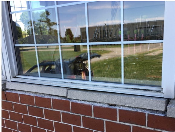
Dislodged precast window sills
